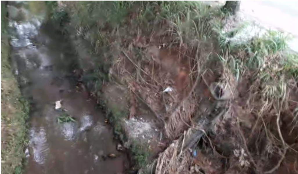
Figure 13. Sewage discharge in natura and erosion
